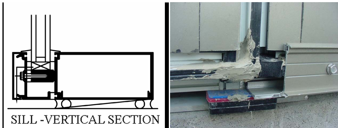
Figure 5. A typical vertical section detail of exterior wall's sill and a photo of the same condition in the field. The front sealant joint is discontinued at every anchor and corner. The back sealant attaches to horizontal mullion which is discontinued at corners and forms gaps at every end. Both sealant beads have insufficient substrate width. The sealant joints, traced 360° around the fenestration perimeter, would typically not withstand the differential movement. The horizontal aluminum leg bridges the mullion thermally. Field-applied systemic sealant separates wet and dry zones of the curtain wall.
